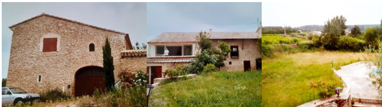
These give a bit of an idea of the state of the place.
